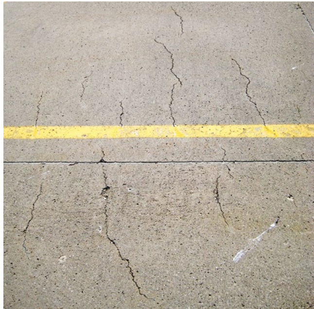
Figure 6-26. Plastic shrinkage cracks
