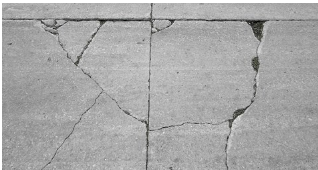
Figure 3-5. Corner cracking in jointed concrete pavement
