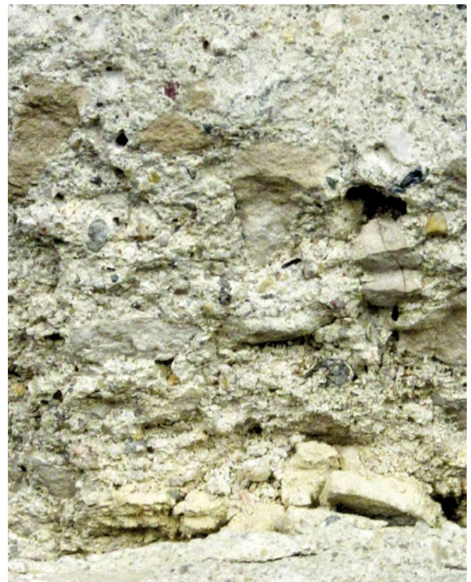
Figure 6-33. Joint damage showing flakes
